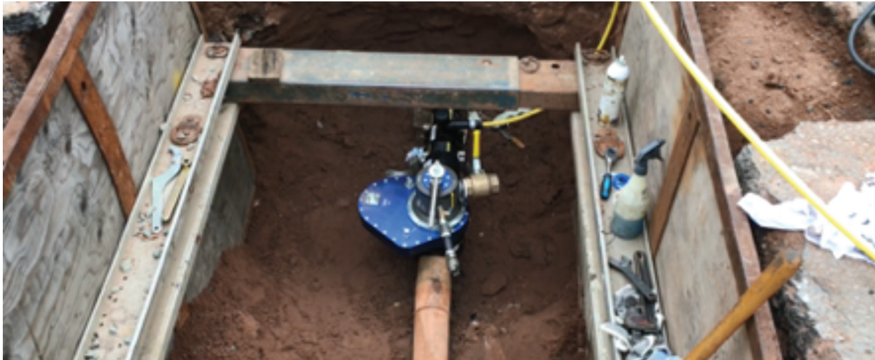
Fig. 1. Line Stopping Performed On a 4" PE Gas Main to Remove an Outdated Pipe Fitting
